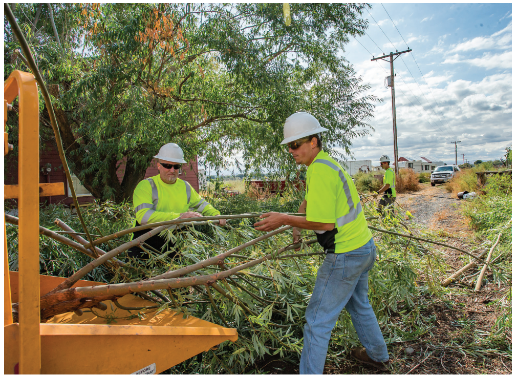
Staff photo by Ben Lonergan/East Oregonian Ricky Parsons, left, and Andy Renoe work to load tree trimmings into a chipper after trimming a tree to avoid a set of power lines off of Agnew Road in Hermiston. Parsons and Renoe are employees of The Tree Service, a company contracted to trim trees for Umatilla Electric Cooperative.
