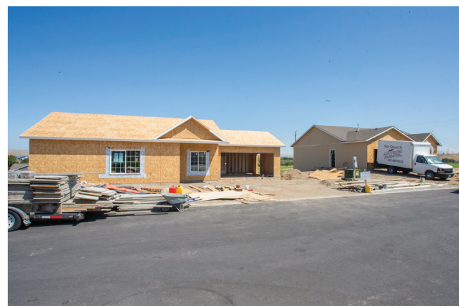
A pair of nearly completed homes undergo construction work in an expanding development in Umatilla.
