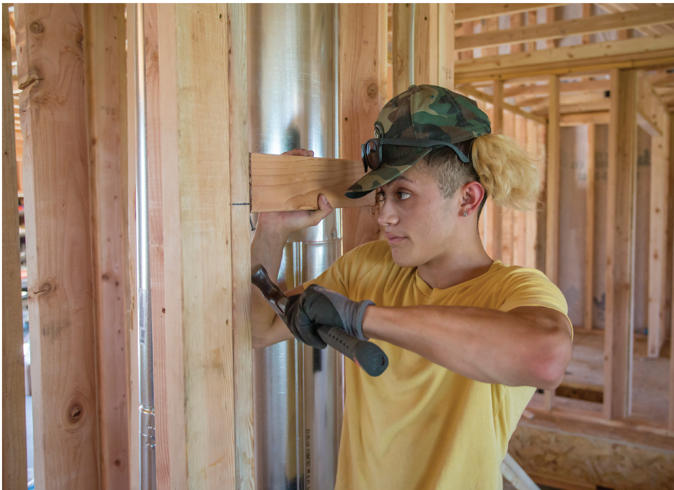
Isaiah Aquilar fastens a 2 by 4 piece of lumber in a new home construction project in Umatilla.
