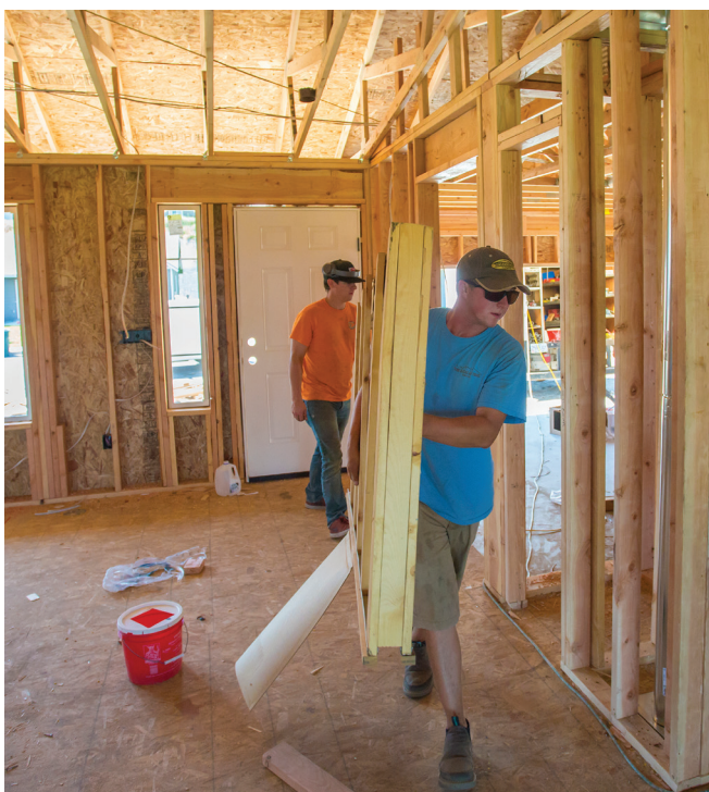
Jacob Edens carries a pocket door frame into a new home construction project in Umatilla Thursday afternoon.
