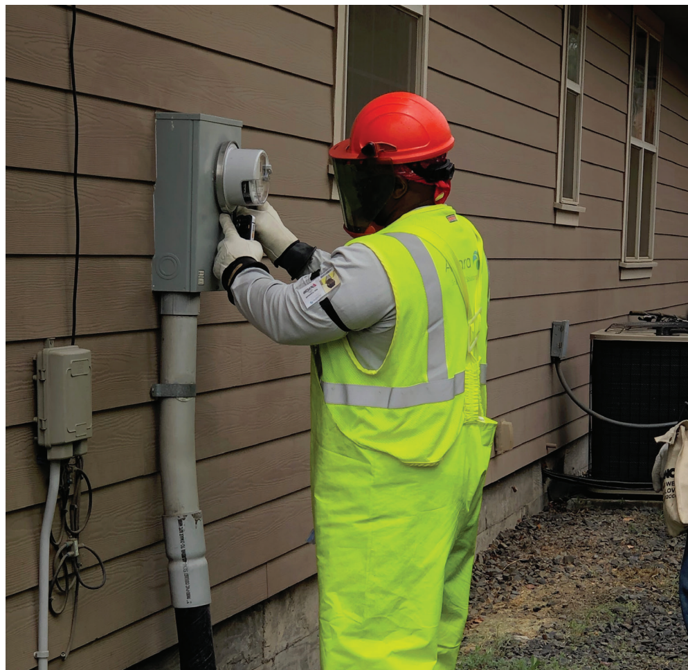
A Pacific Power employee works on a meter at a recent smart meter installation demonstration in Pendleton.
