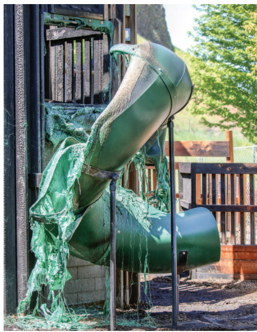
Fire destroyed a play structure early Friday morning at Hermiston's Funland Park, melting this slide.
