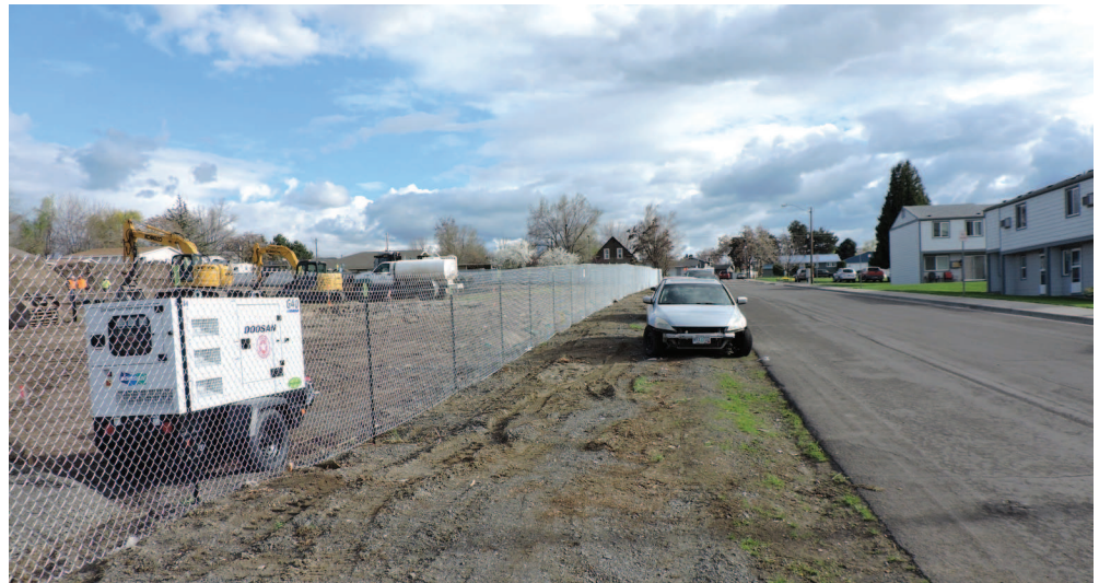
Construction is underway for Hermiston Family Housing, a new 48-unit apartment complex on Southeast Sixth Street across from the Cottonwood Apartments in Hermiston.
