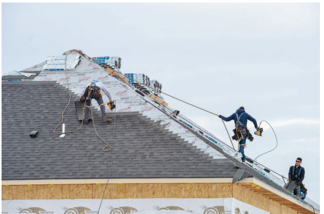
Staff photo by E.J. Harris Roofers work on a home under construction in the Desert Sky Estates on Tuesday in southwest Hermiston.
