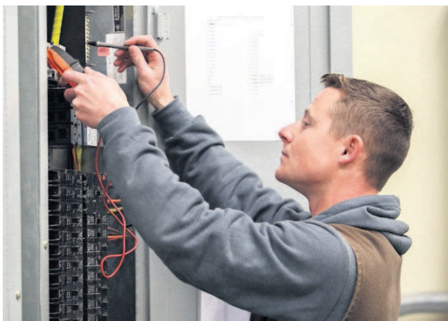
Cody Kile checks the voltage in one of the electrical panels at Good Shepherd Medical Center during time as an electrician apprentice with Gordon's Electric.
