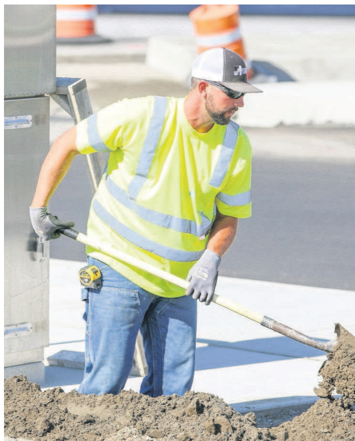
STAFF PHOTO BY KATHY ANEY Josh Ross, of Ross-Brandt Electric in Hermiston, digs a trench near the intersection of 11th Street and Elm Avenue in Hermiston.
