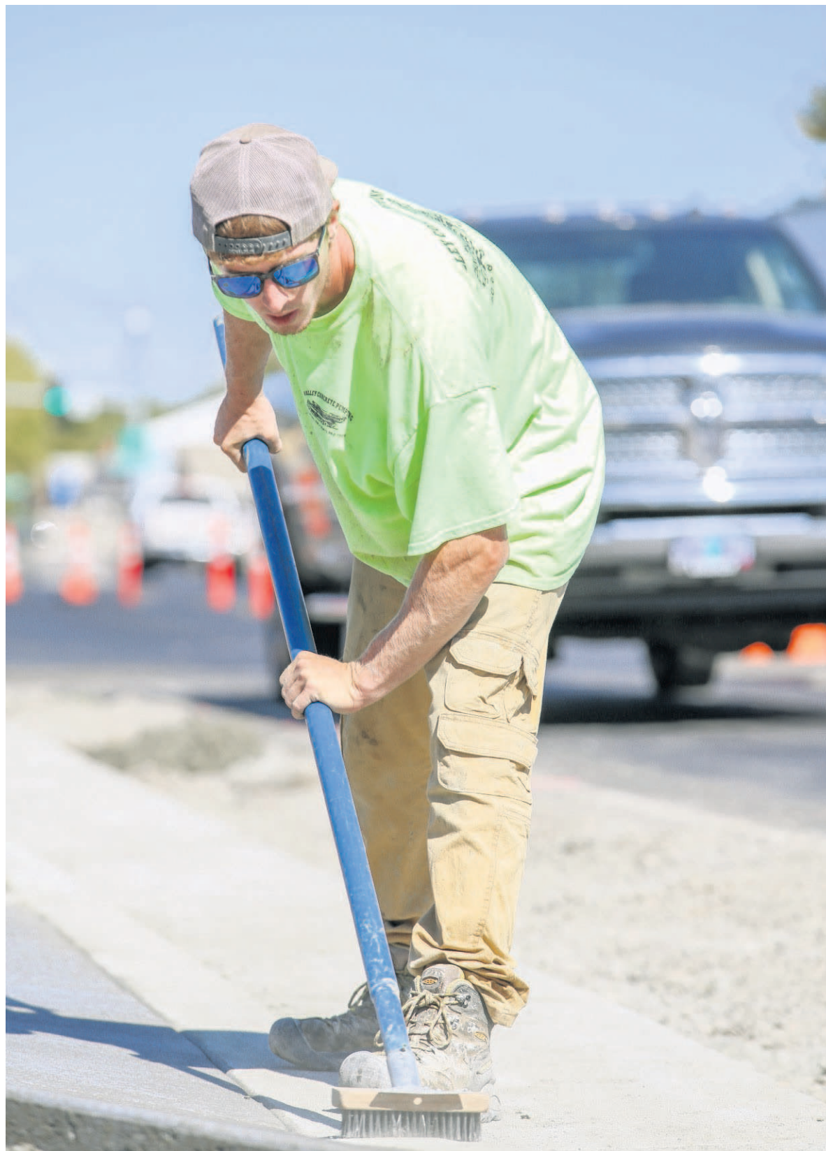
Blue Chavez, of Challis Concrete Construction in La Grande, sweeps some freshly dried concrete Tuesday near the intersection of 11th and Orchard in Hermiston.
