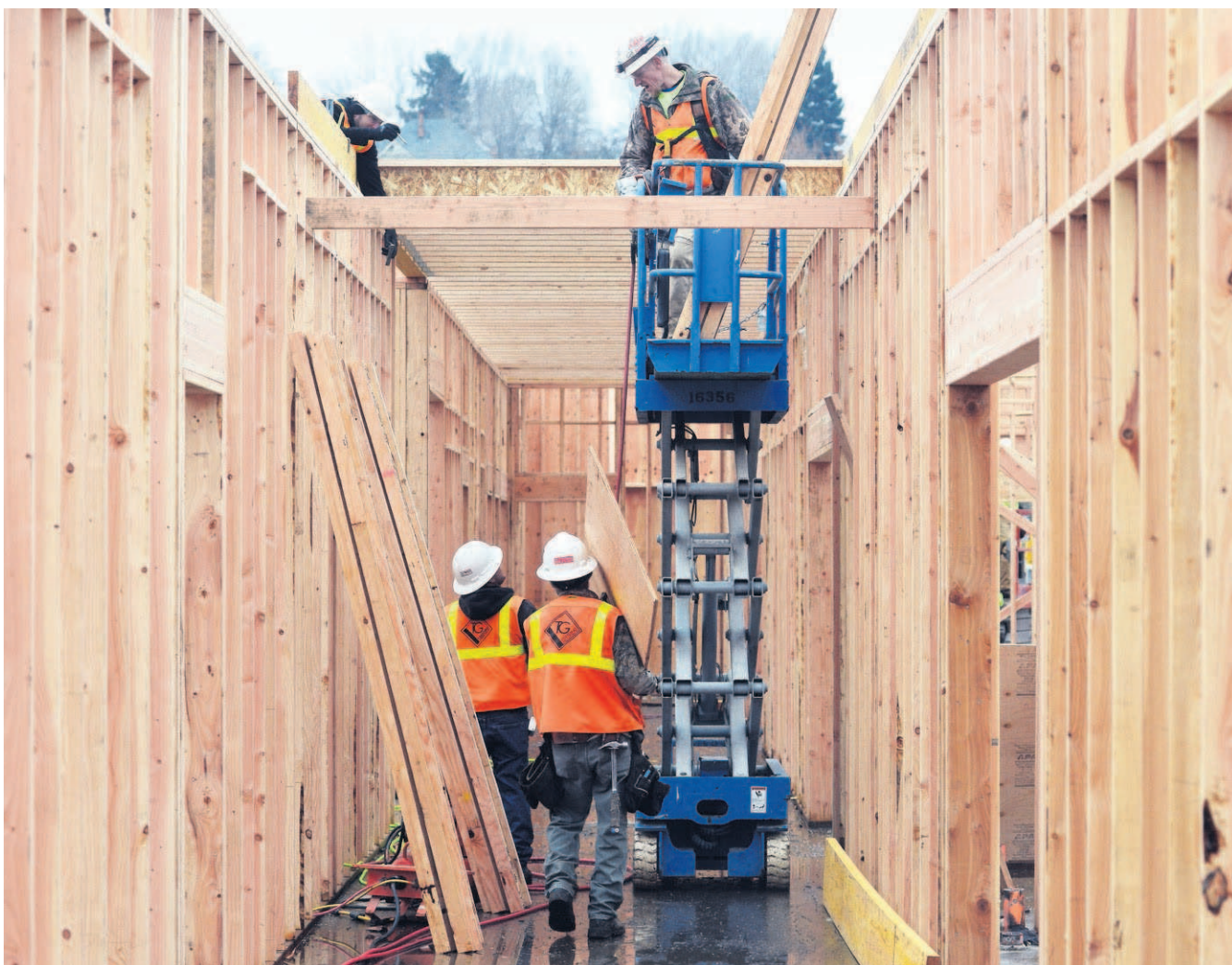
FILE PHOTO BY E.J. HARRIS Construction crews contracted by the Wenaha Group work on the Hawthorne School building in December 2014 in Pendleton. Construction workers and carpenters are among the difficult-to-fill jobs that make up the majority of job vacancies in Eastern Oregon.
