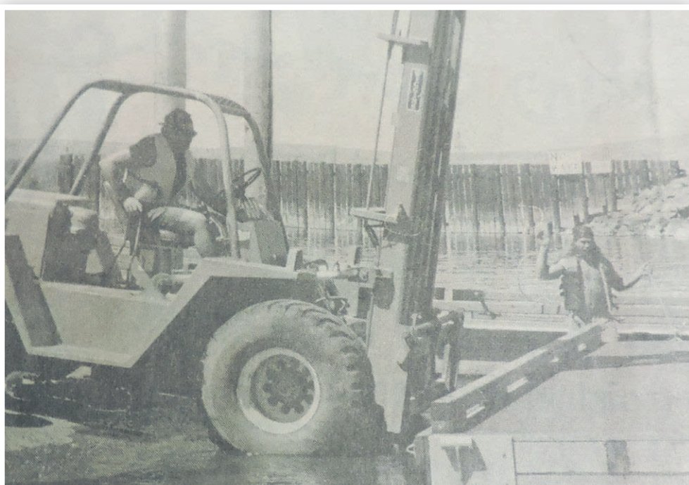
Jon Colon of Knerr Construction lowers a repaired boat launch into the water at the Umatilla Marina, directed by Charlie Dickerson.
