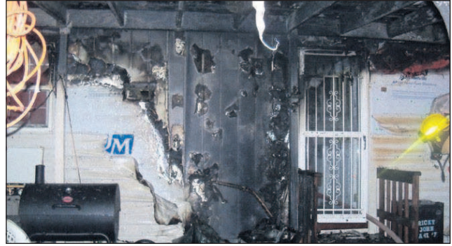
PHOTO CONTRIBUTED BY UMATILLA COUNTY FIRE DISTRICT 1 A fire did serious damage to a house Wednesday morning on Southwest Joseph Avenue in Hermiston.
