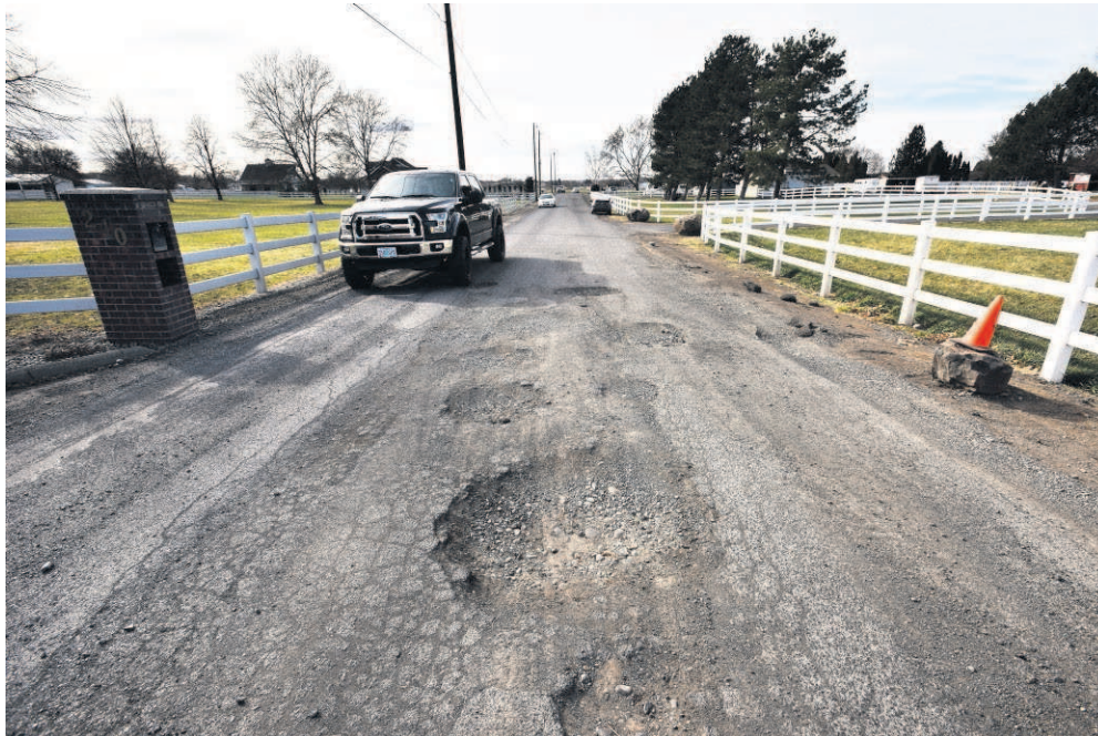
A truck drives around the potholes in the middle of East McKinney Avenue on Tuesday in Hermiston.
