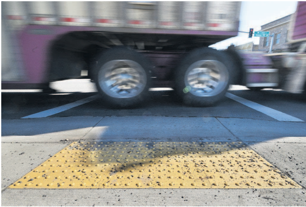
A semi-trailer passes in front of an ADA-compliant wheelchair ramp crossing Highway 395 in Hermiston.
