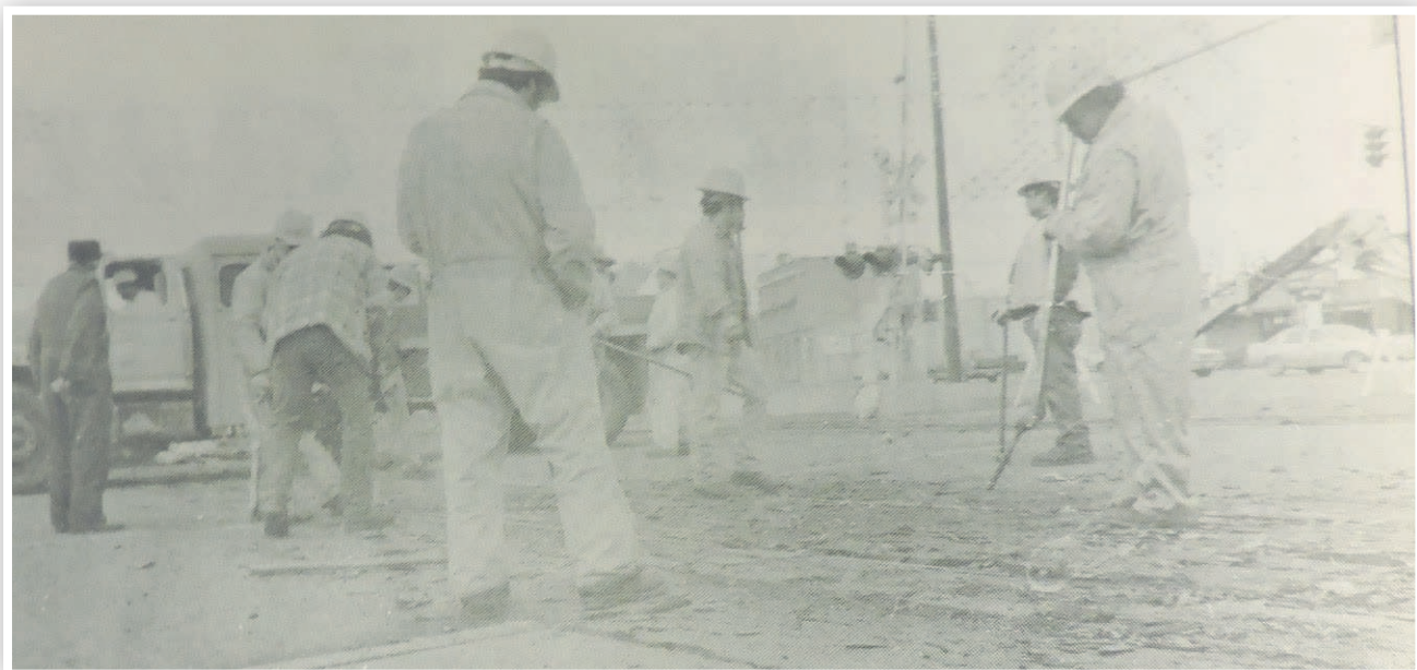
Union Pacific employees replace wooden railroad ties with concrete ones, which will make driving over them less bumpy for vehicles. The construction blocked traffic on Orchard Avenue, in February of 1993.
