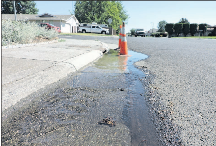
Water flows from a storm drain at the corner of West Division Avenue and Southwest Seventh Street. The water, which has been flowing steadily out of the drain for about a week, has been traveling two blocks down Seventh Street to another drain on Highland Avenue.
