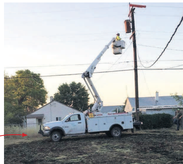
PHOTO CONTRIBUTED BY KIRSTEN WRIGHT A transformer explosion sparked a back yard fire at a home on Ridgeway Ave. in Hermiston on Monday.
