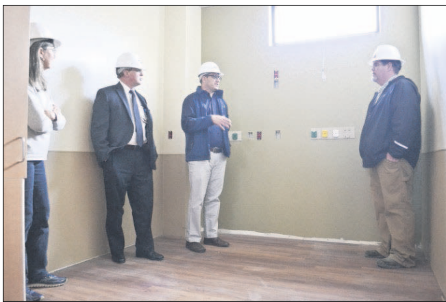
Chris Giles, right, project superintendent from McCormack Construction Company, tasked with completing the surgical expansion at Good Shepherd Medical Center, talks with community members and Kelly Sanders, GSMC vice president of human resources, second from left, about the improvements GSMC's surgical wing will have.
