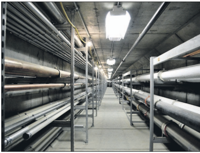
Pipes that allow flow of steam, electricity, oxygen and other surgical gases will run through a tunnel under ground that will flow from the hospital's new surgical supply building to the surgical wing and the rest of the hospital.
