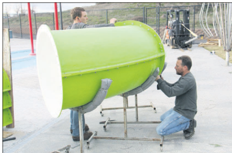
Adam Cornelius, left, and Josh Cornelius, subcontractors for slide company AquaBlue, bolt pieces together for the new slide at the Hermiston Family Aquatic Center Thursday.
