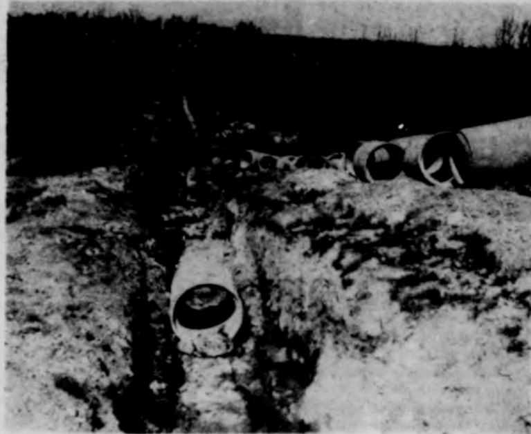
Pictured above is the break in the K irrigation line which has caused a delay in getting water to the east side of Hermiston. The break has now been repaired and water will flow this week end.
