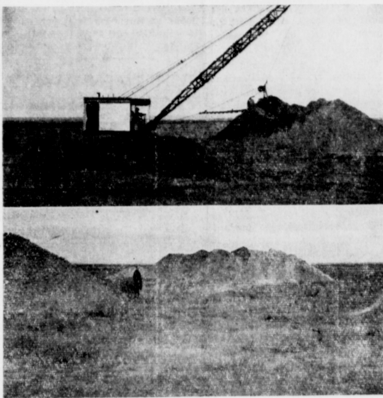
Pictured above is a drag line at work digging test holes at the site of the Umatilla Ordnance Depot. Work was started Tuesday on these test pits as well as grading for roads. The lone sentinel in the lower picture is none other than the sage of Hermiston, E. P. Dodd. Photo G. Felthouse
