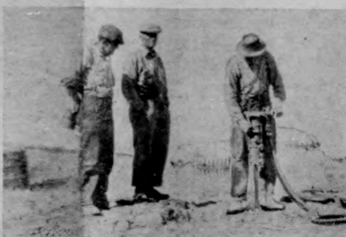
The first hole drilled in the construction of the 8.3 miles of highway on the Wallula cut-off Sand Station at State Line highway about June 3. Mr. Parker, foreman on the job, is pictured standing in the center. Two miles of grading has been completed since that time.
