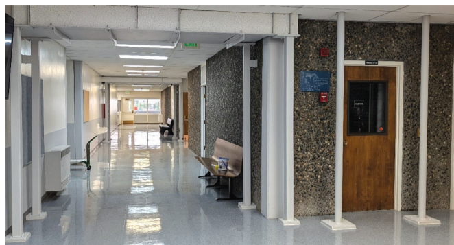
Pictured is the shoring work that was completed in the main hallway at Irrigon Jr Sr High during December 2023.
