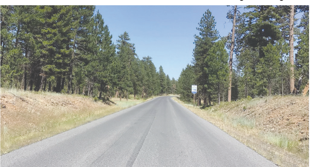
Photo of completed chip seal on the Blue Mountain Scenic Byway. -Contributed photo
