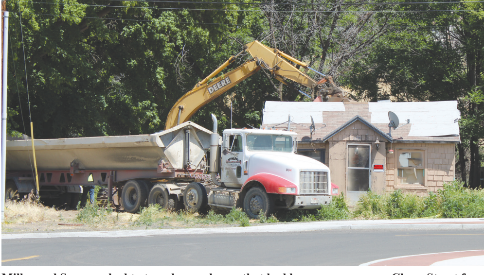
Miller and Sons worked to tear down a house that had been an eyesore on Chase Street for many years. - Photo by Andrea Di Salvo
