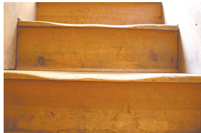
Stairs worn down by five generations of Wright feet. -Photo by Andrea Di Salvo
