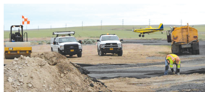
The Morrow County Airport in Lexington is slated to receive more than $200,000 in Dept. of Transportation infrastructure grants for runway improvements. -Contributed photo
