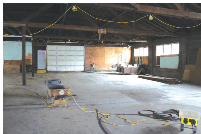
Toward the back of the building will be an L-shaped event area, separated by breakfast bar from a certified kitchen. A roll-down door over the bar will allow the two spaces to be separated. The roll-up door in the back will remain—in a way. It will be replaced by a glass rolling door and will open onto a patio area edged by a retaining wall. -Photo by Andrea Di Salvo
