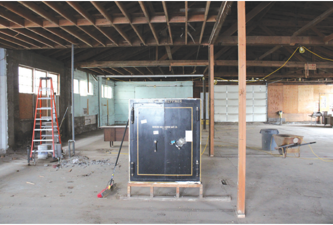
Visitors will hardly recognize the former Gazette-Times office. Gutted right now, it will become a cluster of offices and a center for business services and training. -Photo by Andrea Di Salvo
