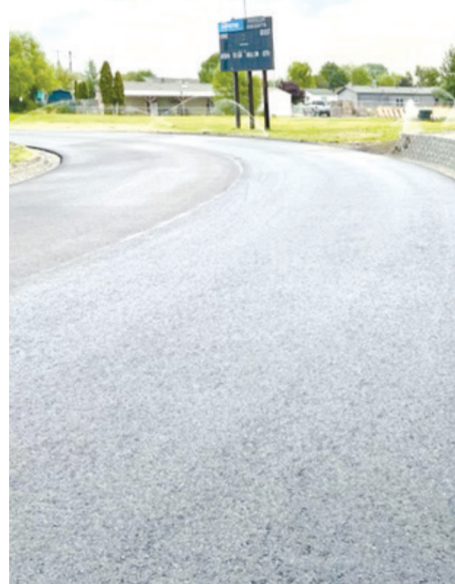
Currently, there is a three-inch deep base layer of asphalt, which will be covered in the next phase with a synthetic rubberized surface.
