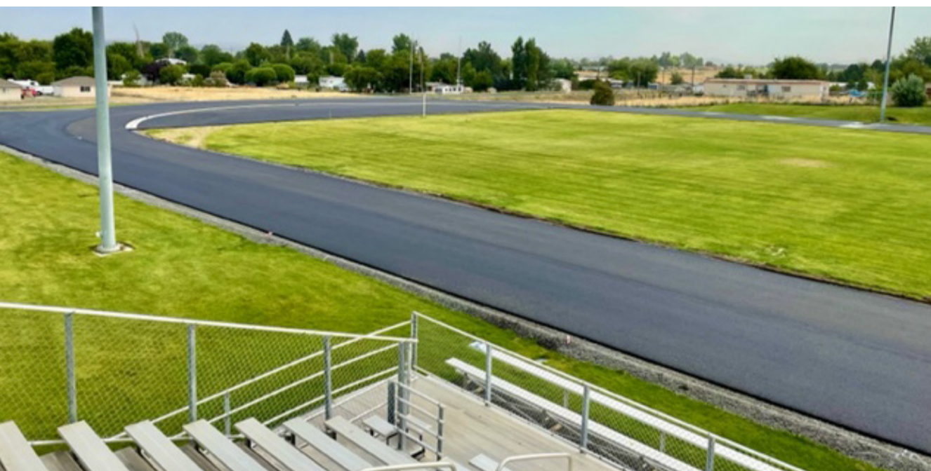
One big improvement is the new track currently under construction at Irrigon Junior-Senior High.
