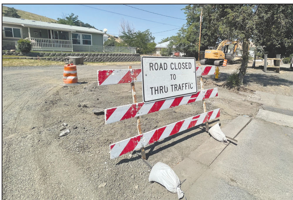
Work crews were busy on Jones St this past week. -Photo by Chris Sykes
