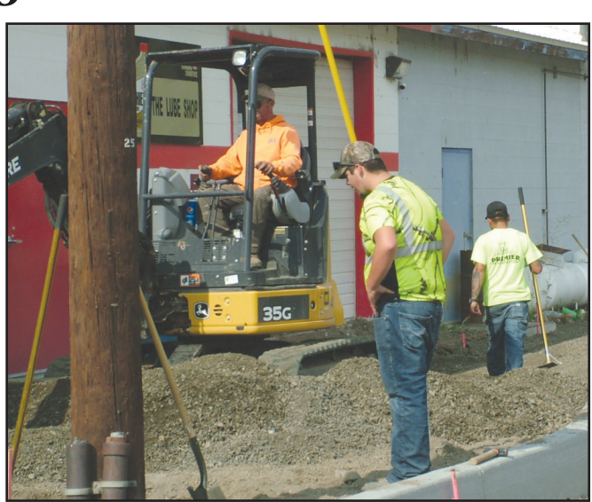
Work continued this week on the big Heppner renovation street project, which city manager Kraig Cutsforth says is on schedule to be completed by November. -Photo by Hannah Finch
