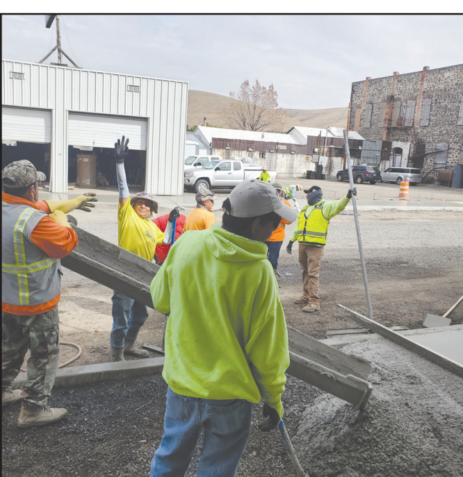
The crew putting in Heppner's new curbs and sidewalks was back in town and on the job last week. They started at the north end of Gale Street (right) and also did work on Willow (left). The company had been gone for a week waiting for preparation work to be completed before they could start pouring concrete. "They move pretty fast," said city manager Kraig Cutsforth commenting on the progress. The curbs and sidewalks are part of the bigger street renovation going on in Heppner, and when sidewalks are completed the pavers will then be coming in to complete the renovation.
