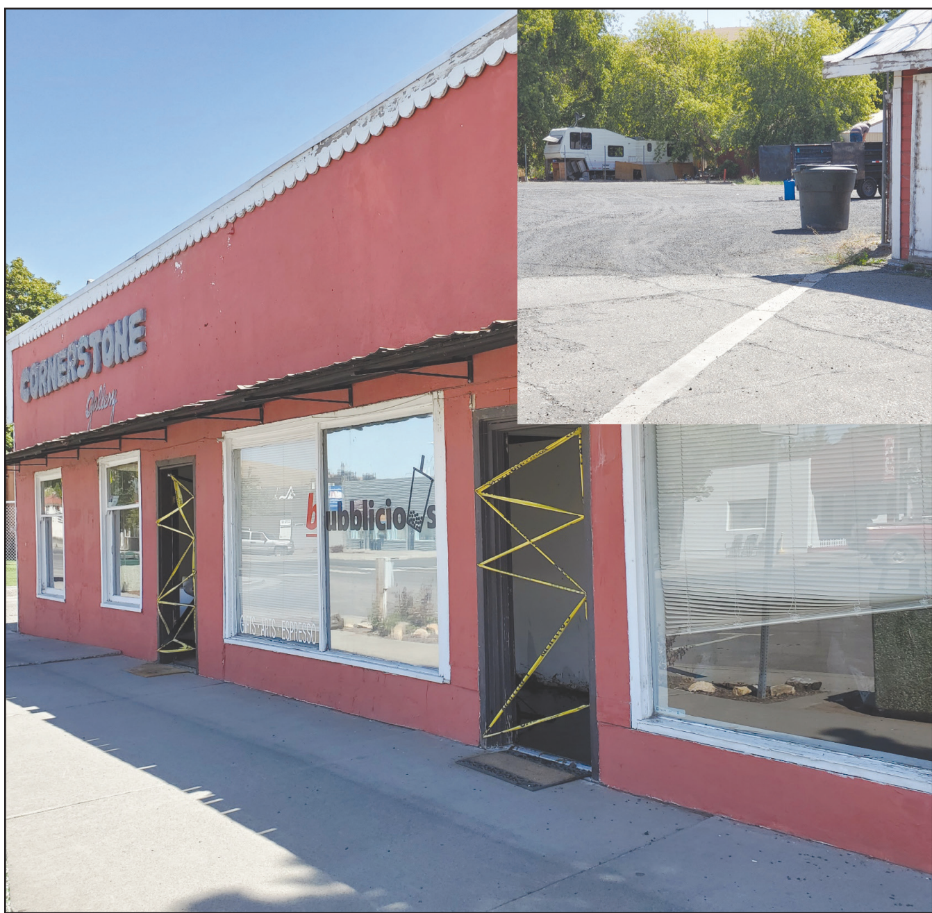
Sale of this Main Street property has been completed and construction of a new Dollar General store will now begin in Heppner. Monday workman were already inside the former Cornerstone Gallery building, and the former RV park now sits empty of trailers (inset). -Photo by David Sykes.
