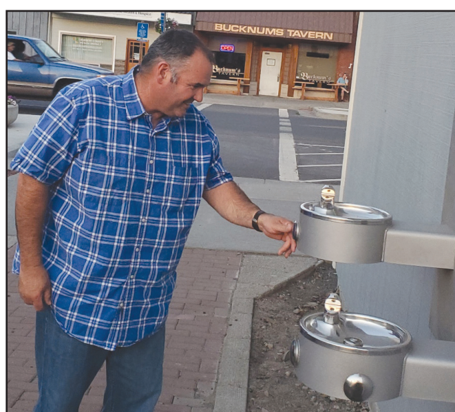
Heppner City Council member Corey Sweeney inspects new water fountain being installed at Thompson Square Food Court. -Photo by David Sykes
