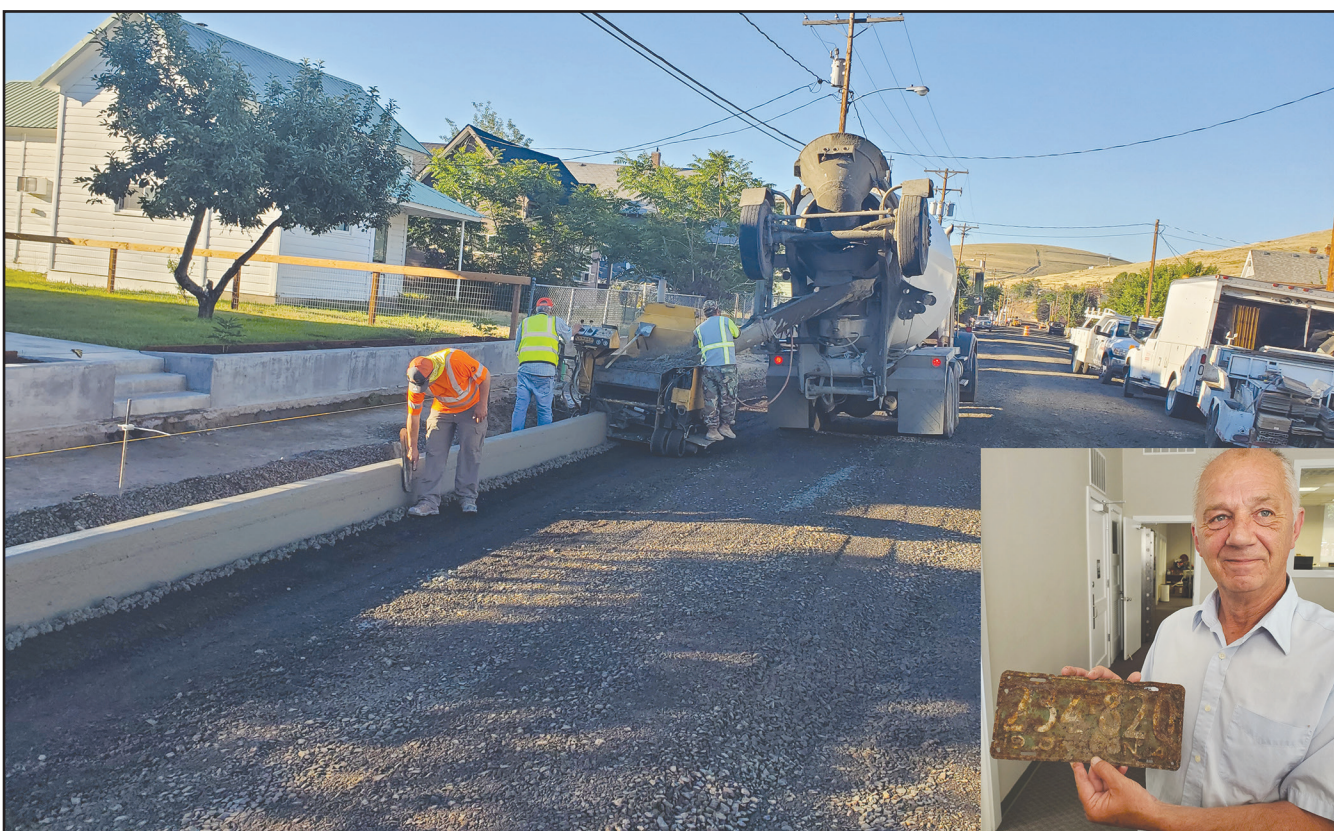
Workers began installing curbs and sidewalks Tuesday on the north end of Gale Street. The crews will be starting at 5 a.m. to beat the heat. Where were you in 1941? Heppner City Manager Kraig Cutsforth (inset) holds a 1941 automobile license plate uncovered during the street renovation project now going on in Heppner. Cutsforth says nothing too "unusual" has been unearthed during the renovation project. -Photos by David Sykes
