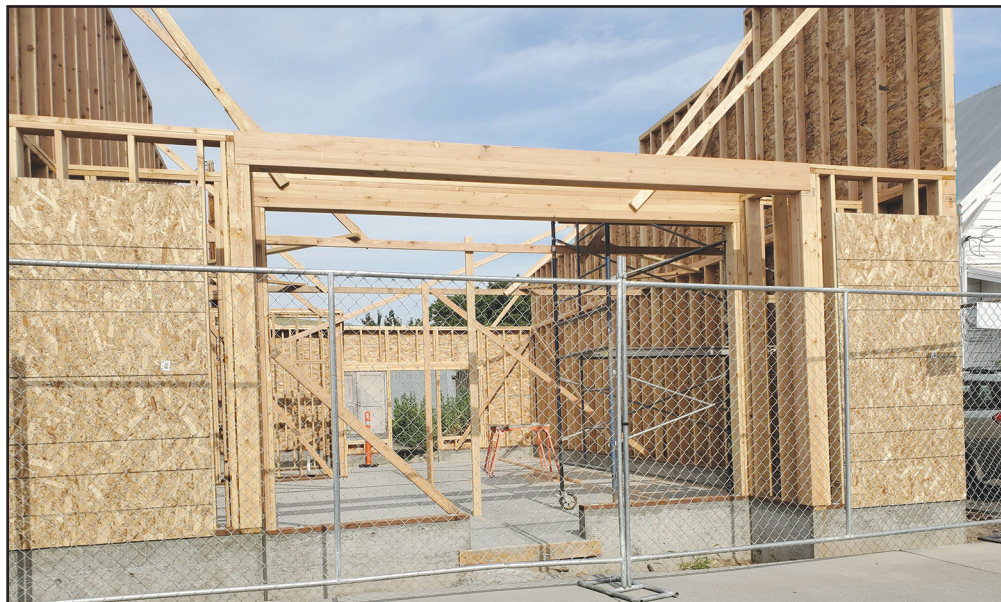
Now under construction is the new "Lotts of Fitness" workout center on Main St. -Photo by David Sykes
