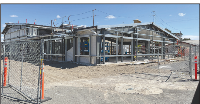
Construction is moving along on the new county office building complex in Irrigon. -Photo by Chris Sykes.
