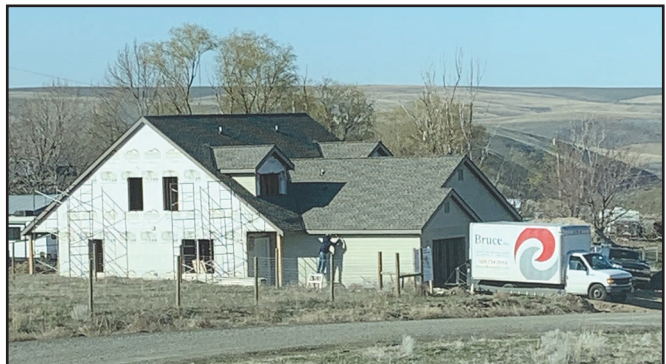
The new duplex is being constructed at the top of the Emert 2 subdivision.
