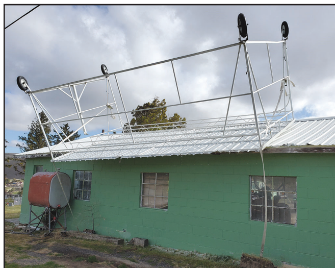
High winds picked up the mobile shade structure at the Heppner cemetery and deposited it on top of the shop building. -Photo by Giselle Moses.
