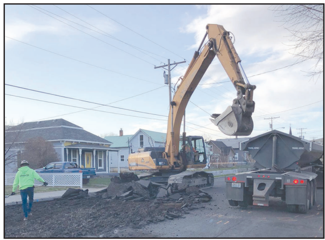
Backhoes began tearing up and removing the pavement on Chase Street last week in preparation for the new street to be put in. -Photo by Tripp Finch
