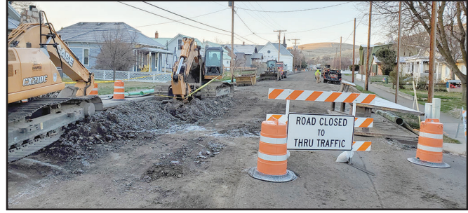
Things will be a little rough on some streets in Heppner for the next several weeks as the city completes a badly needed rehabilitation project. -Photo by David Sykes
