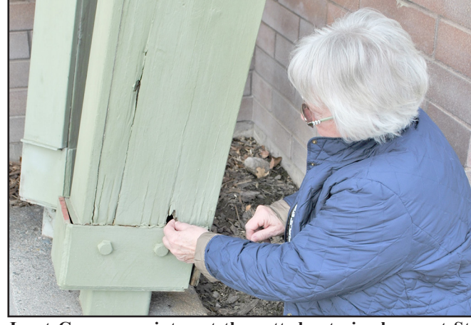
Janet Greenup points out the rotted exterior beam at St. Patrick's.
