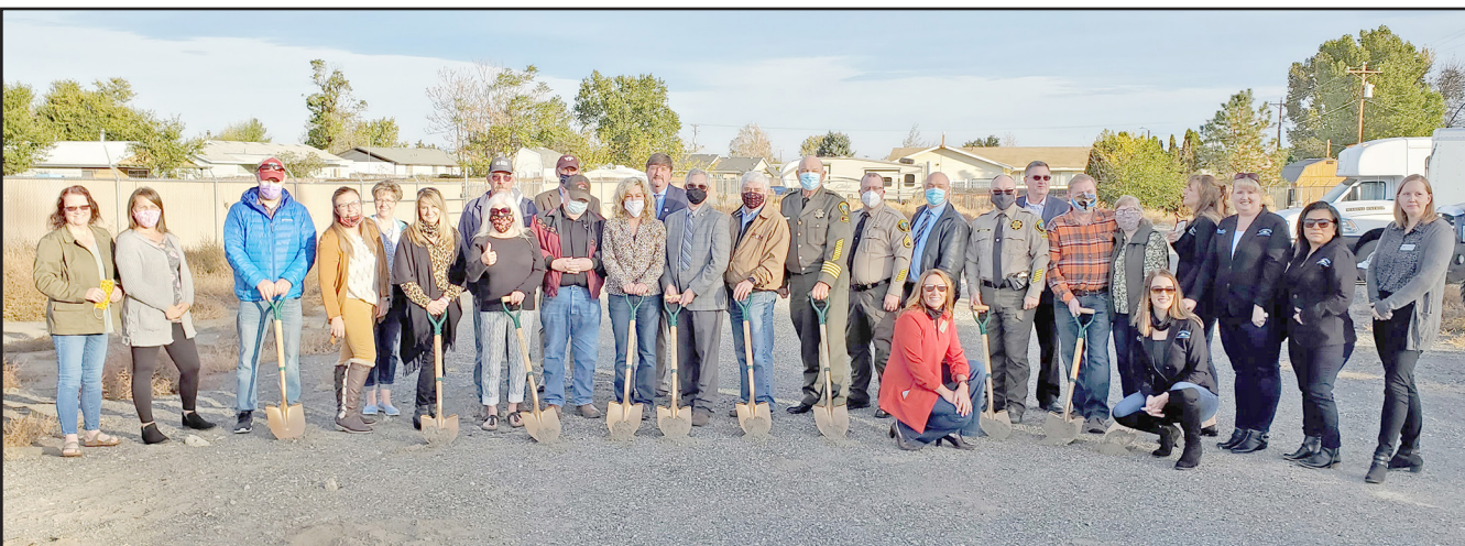
A large group of county and city leaders and staff gathered last week for the groundbreaking of the new county administrative building in Irrigon. -Photo by David Sykes
