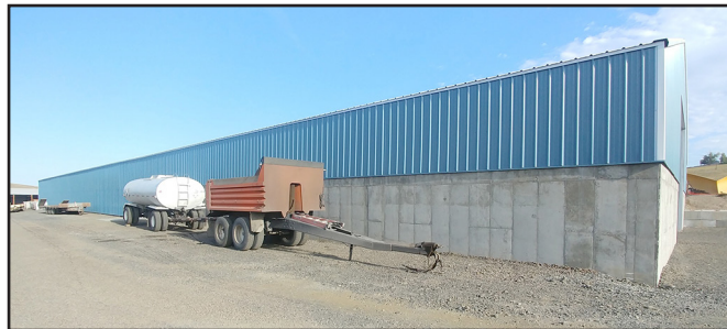
Morrow County Public Works has been building a new storage facility in Lexington. One end will be for equipment storage and the other end will store sand. -Photo by Bobbi Gordon.
