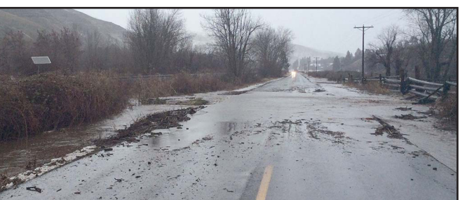
Photo of standing water on road near Gibbon, Oregon, taken Feb. 6, 2020.
