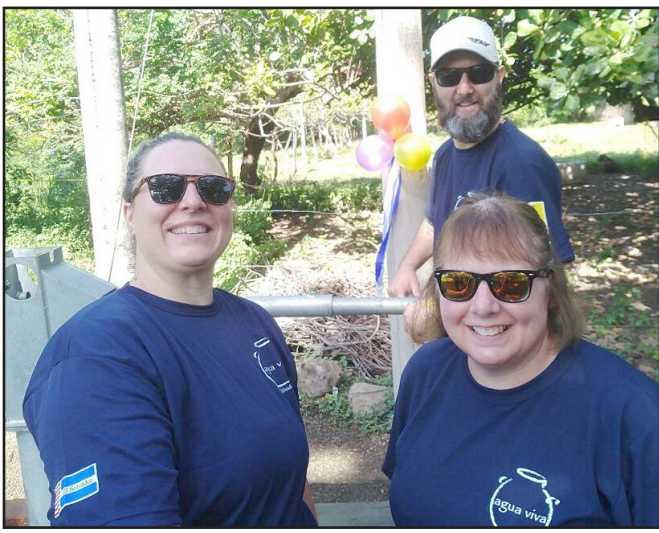
Danny Sharp, Katie Fuller and Vicky Rayburn work on a well drilling project in El Salvador.
