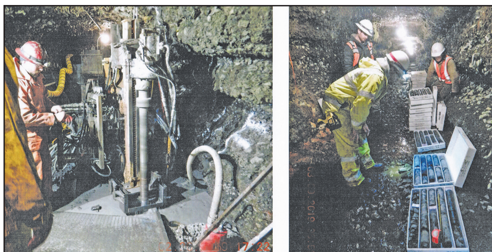
Workers drill into the Willow Creek Dam taking core samples for study. The drilling is part of the periodic inspection of the dam and was done in February and March of this year.
