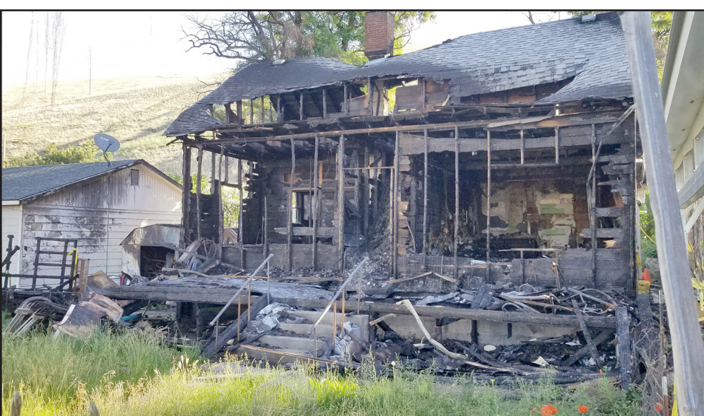
This house on 485 Linden Way was gutted by fire April 2. Over two months later it still has not been removed. -Photo by David Sykes.
