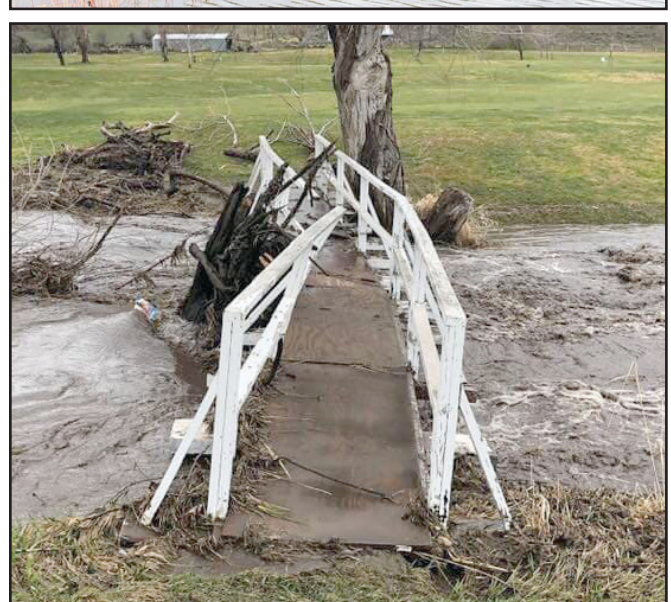
The footbridge at the golf course was damaged by flood waters from Willow Creek.
