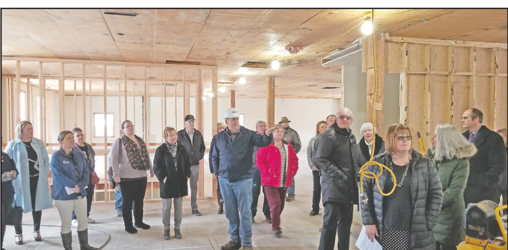
Local contractor David Allstott (center) explains the work going on upstairs at the Gilliam Bisbee building to a group of Chamber of Commerce members. -Photos by David Sykes.
