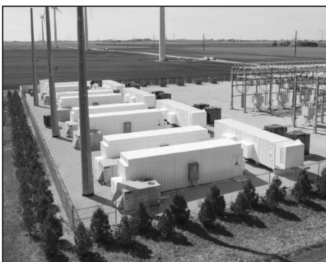
If a revised wind farm plan is approved by the state, a battery energy storage facility like this one will be built in Morrow County. The facility has 3,000 batteries and stores power generated from the wind towers.
